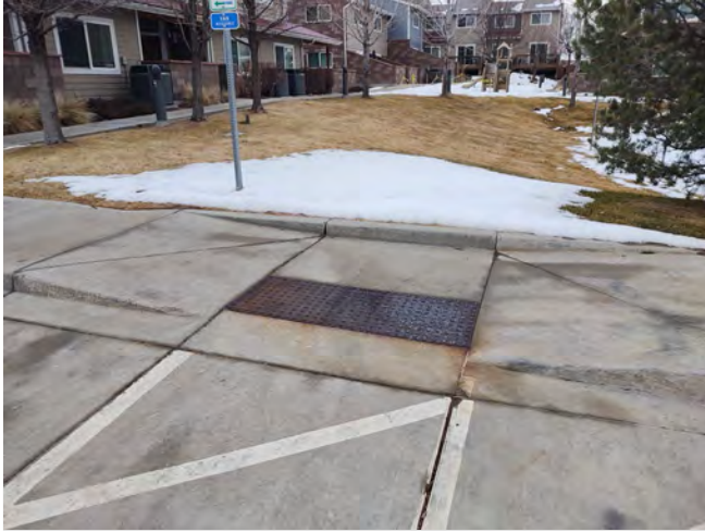
Photo AMN1 – Curb ramp at accessible parking space at west end of complex.
