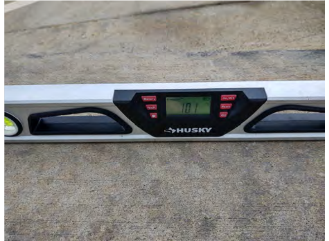
Photo AMN2 – Running slope on one side of curb ramp at 10.1%.
