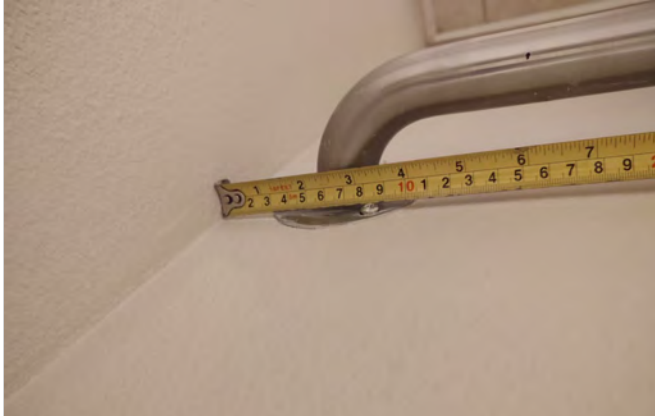
Photo AMN9 – Dwelling Unit C6 - Measured dimension to near edge of rear grab bar at 3” from the side wall.
