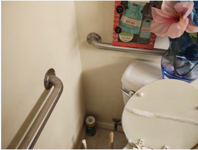
Photo AMN5 – Dwelling Unit C1 - Flush control on wall side of water closet.
