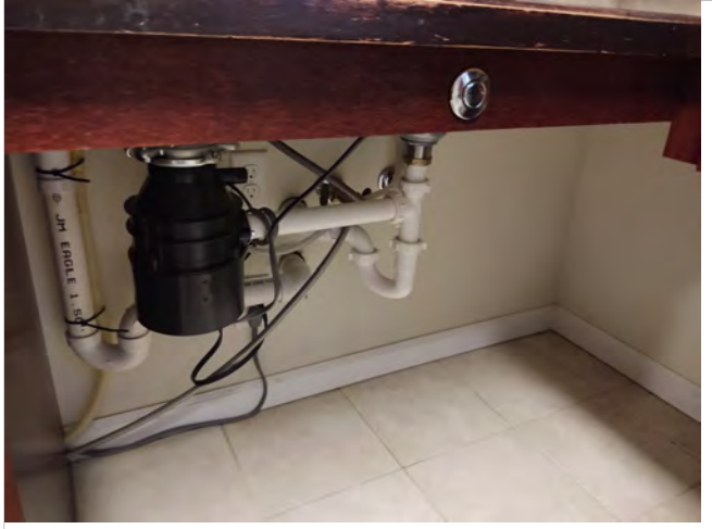
Photo AMN11 – Dwelling Unit C6 - Exposed piping beneath kitchen sink.
