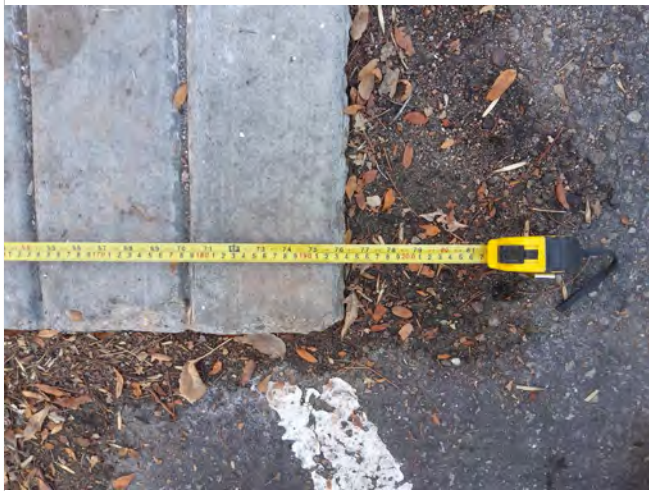
Photo CS3 – The curb ramp extends 76” into the access aisle.
