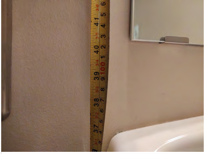
Photo CS5 – Unisex Toilet Room – Measured height of 40 ½” to bottom of reflective edge of mirror.
