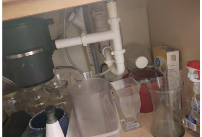
Photo L10 – Community Room – Exposed piping beneath kitchen sink.
