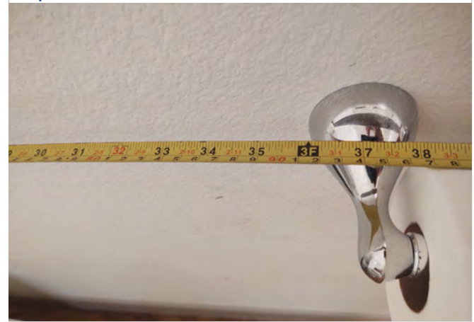
Photo L20 – Dwelling Unit #106 - Measured dimension of 37” to front edge of toilet paper dispenser.
