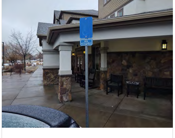
Photo L2 – Faded accessible parking signage
