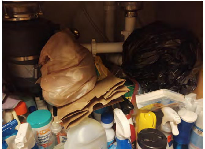
Photo L18 – Dwelling Unit #104 - Exposed piping beneath kitchen sink.
