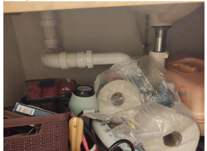
Photo L16 – Dwelling Unit #104 – Exposed piping beneath bathroom sink.
