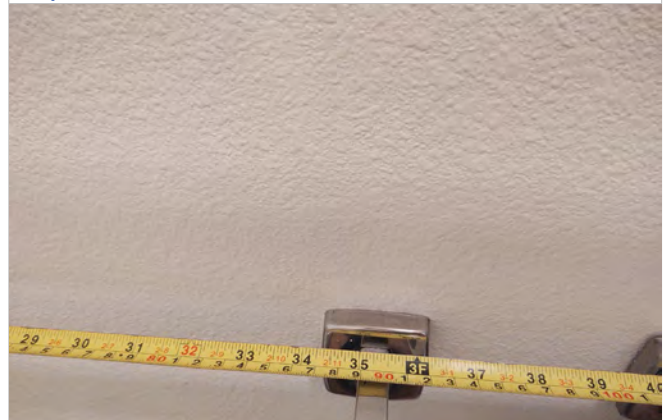
Photo L14 – Dwelling Unit #104 – Measured dimension of 36” to front edge of toilet paper dispenser.
