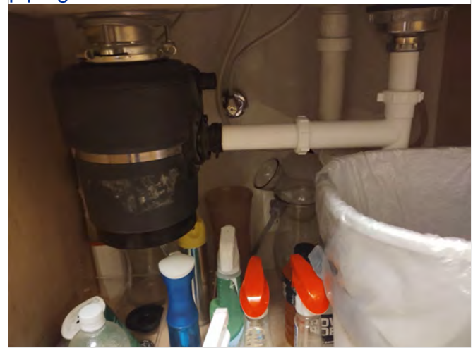
Photo L24 – Dwelling Unit #106 - Exposed piping beneath kitchen sink.
