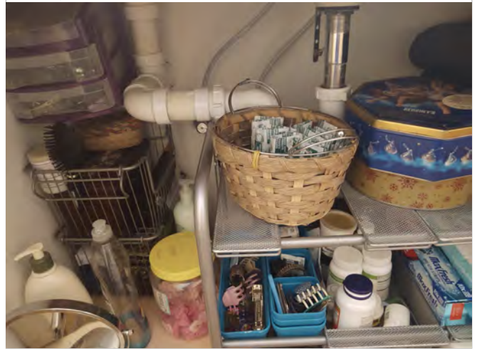
Photo L22 – Dwelling Unit #106 - Exposed piping beneath bathroom sink.
