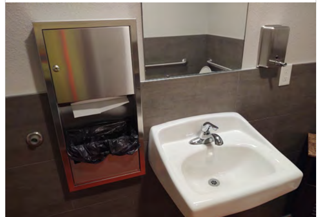
Photo SC16 – Second Floor Unisex Toilet Room – View of mirror over sink that exceeds 40”.
