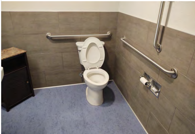
Photo SC17 – Third Floor Unisex Toilet Room - View of toilet paper dispenser that exceeds 36".
