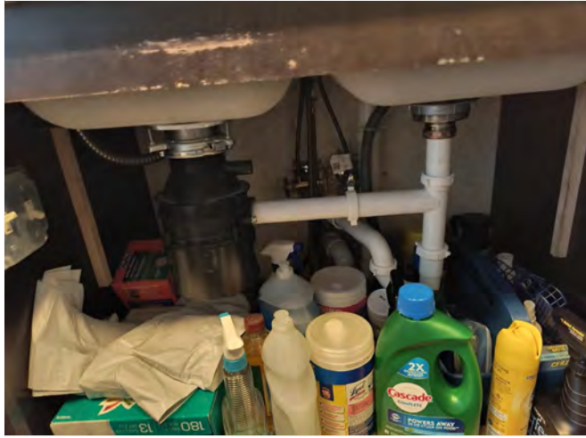
Photo SC24 – Dwelling Unit #309 - Kitchen sink with exposed piping.
