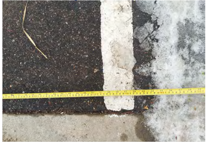
Photo SC6 – Measured width of 50” at access aisle at east wing.
