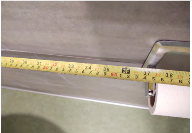
Photo SC11 – First Floor Unisex Toilet Room – Measured dimension greater than 36" to toilet paper dispenser.
