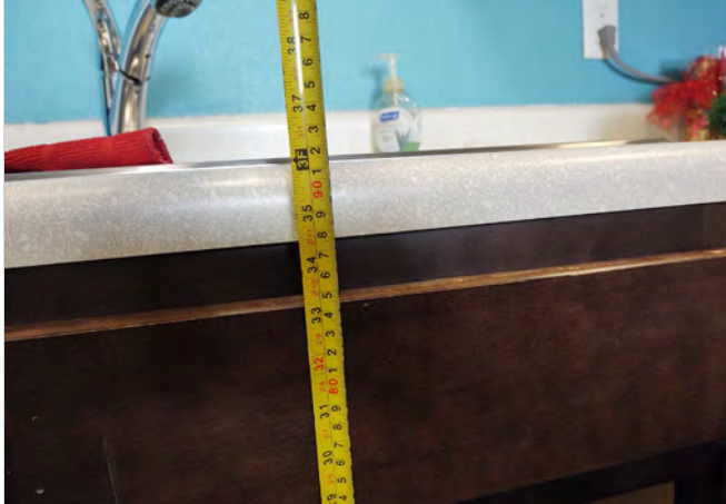
Photo SC9 – Community Room - Measured height of 36" to top of sink.
