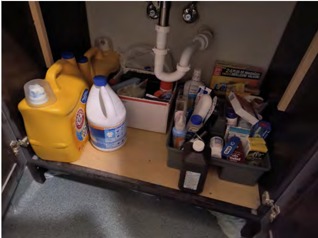
Photo SC23 – Dwelling Unit #309 - Bathroom sink with exposed piping.
