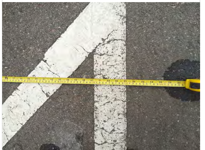
Photo SC4 – Measured width of 49" at access aisle near front entrance.
