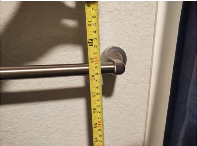
Photo SC22 – Dwelling Unit #212 - Measured height of 59" to towel rack.
