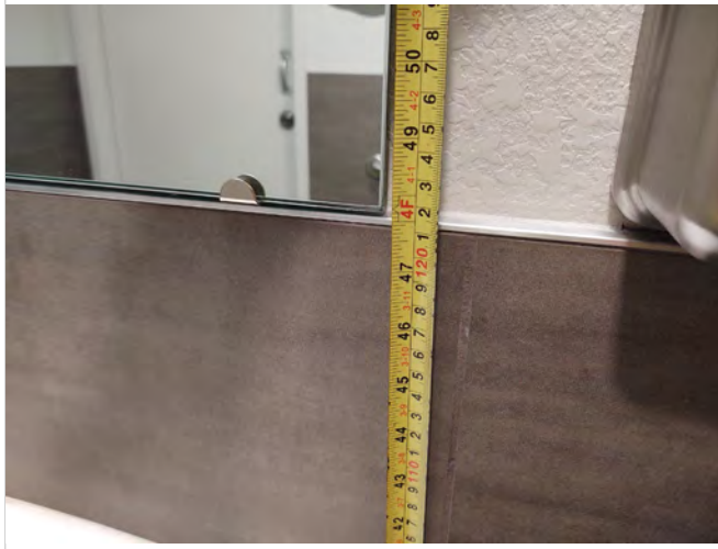
Photo SC13 – First Floor Unisex Toilet Room – Measured height of 48” to bottom reflective surface of mirror.
