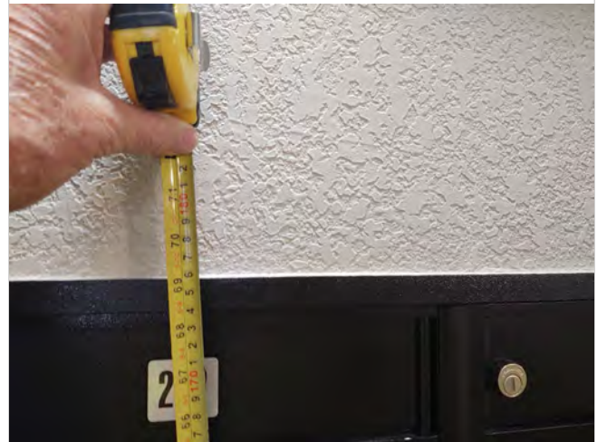
Photo SC8 – Measure height of 68” to top of mailbox bank.
