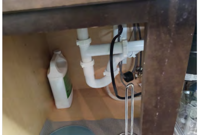
Photo SC10 – Community Room – Kitchen sink with exposed piping.
