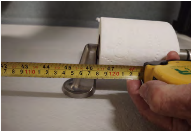
Photo SC21 – Dwelling Unit #212 - Measured dimension greater than 36" to toilet paper dispenser.
