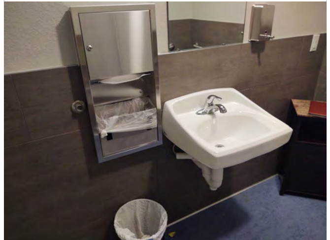
Photo SC18 – Third Floor Unisex Toilet Room - View of mirror over sink that exceeds 40".
