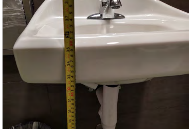
Photo SC14 – First Floor Unisex Toilet Room – Measured height of 35” to top of sink.
