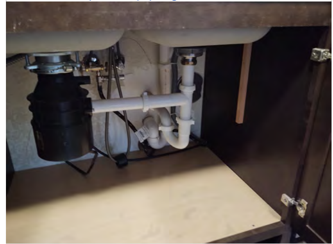
Photo SC20 – Dwelling Unit #119 - Kitchen sink with exposed piping.
