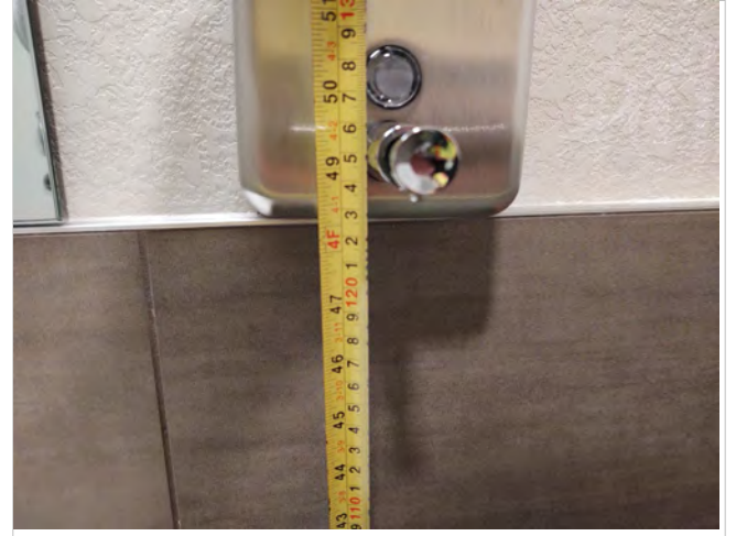
Photo SC12 – First Floor Unisex Toilet Room – Measured height of 49" to soap dispenser.
