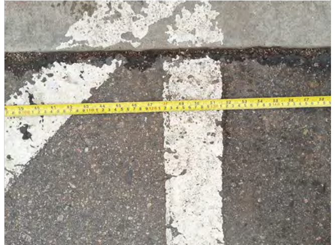
Photo SC2 – Measured width of 50" at access aisle at south wing.
