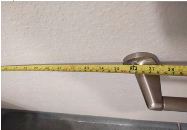
Photo SC19 – Dwelling Unit #119 - Measured dimension greater than 36" to toilet paper dispenser.
