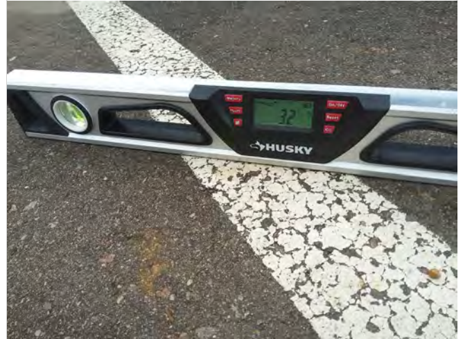
Photo FR2 – Measured slope of 3.2% at accessible parking space.
