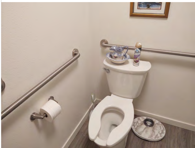
Photo FR19 – Dwelling Unit #207 - Flush control on wall side of water closet.
