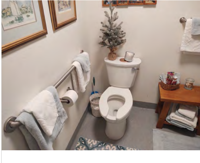
Photo FR15 – Dwelling Unit #107 – Bathroom with no rear grab bar.
