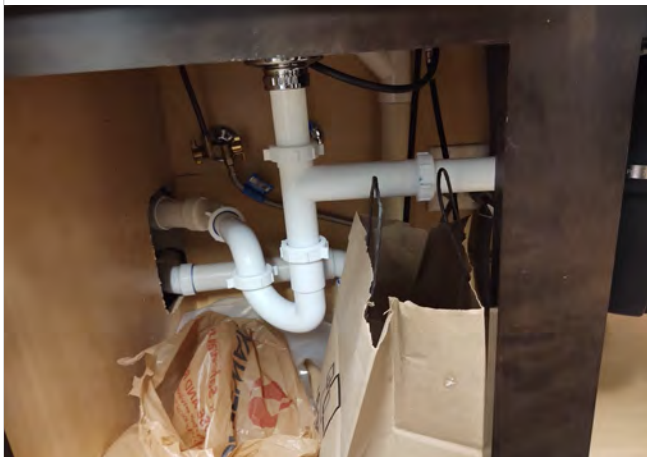
Photo FR7 – Community Room – Kitchen sink with exposed piping.
