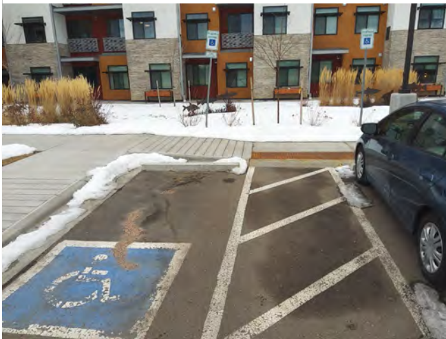
Photo FR3 – Curb ramp on accessible route to front entrance.
