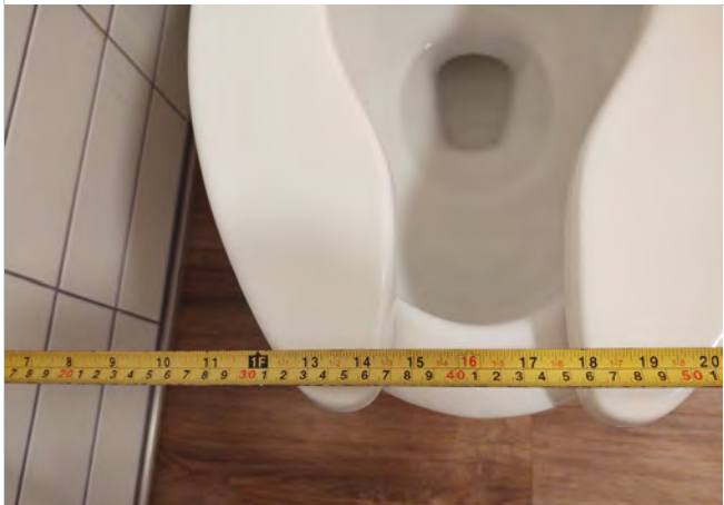
Photo FR11 – Third Level Unisex Toilet Room - Measured dimension of 16 ½” to centerline of water closet.
