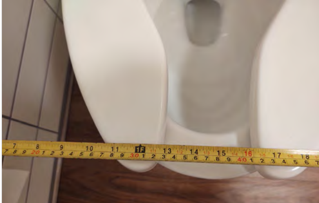
Photo FR9 – Second Level Unisex Toilet Room – Measured dimension of 15” to centerline of water closet.
