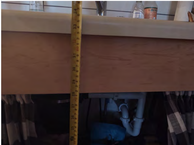
Photo FR17 – Dwelling Unit #107 - Exposed piping beneath kitchen sink.
