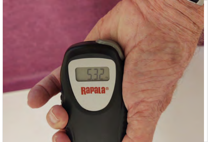
Photo FR14 – Third Level Laundry Room – Measured door pull or 5.32 lbs.
