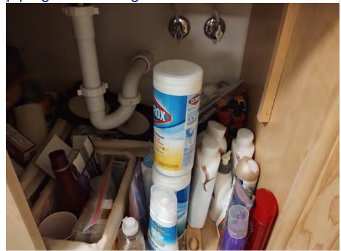
Photo FR20 – Dwelling Unit #207 - Exposed piping and flooring beneath bathroom sink.
