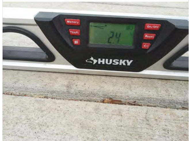
Photo FR4 – Measured cross slope of 2.4% at curb ramp on accessible route to front entrance.
