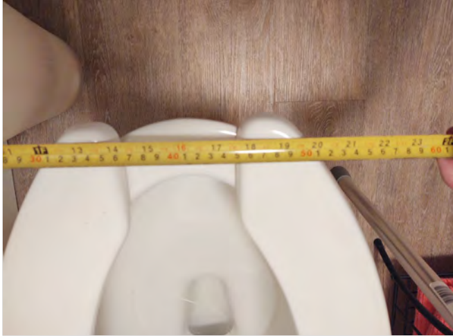
Photo FR25 – Dwelling Unit #414 - Measured dimension of 16" to centerline of water closet.
