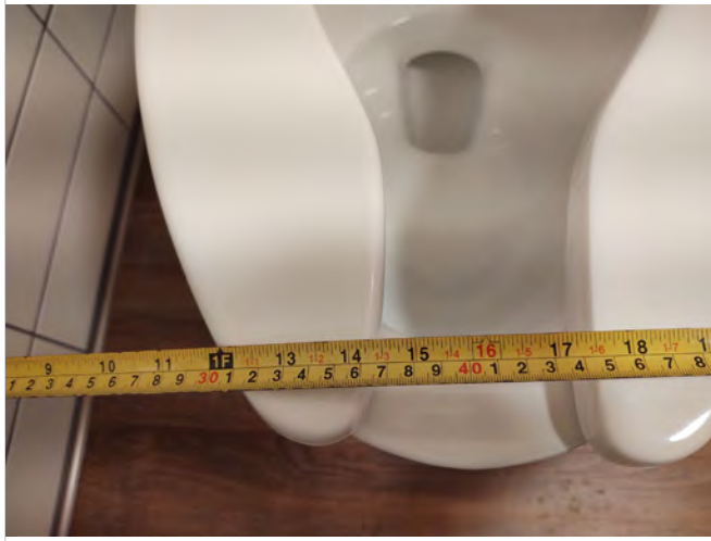
Photo FR13 – Fourth Level Unisex Toilet Room - Measured dimension of 16" to centerline of water closet.
