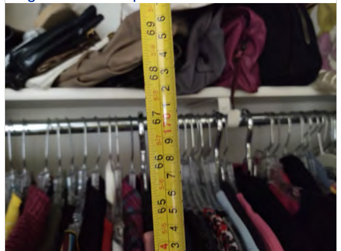
Photo AM8 – Dwelling Unit #104 – Measured height of 67” to top clothes rod.
