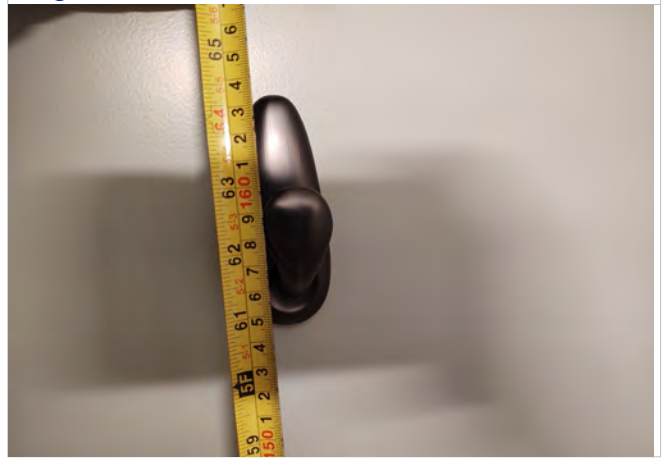
Photo AM6 – Unisex Toilet Room – Measured height of 62” to coat hook.
