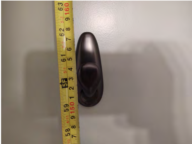
Photo AM7 – Women’s Toilet Room – Measured height of 60” to coat hook.
