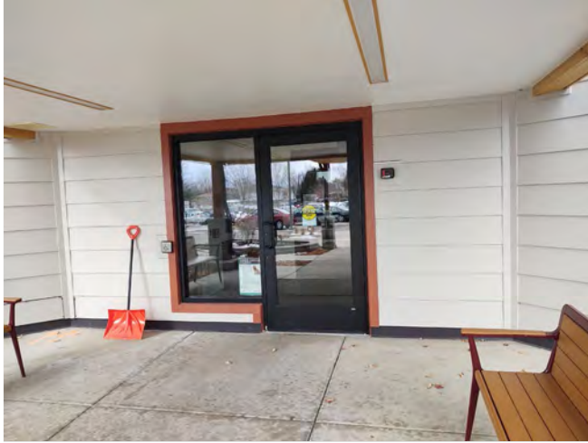
Photo AM1 – Front accessible entrance without signage.
