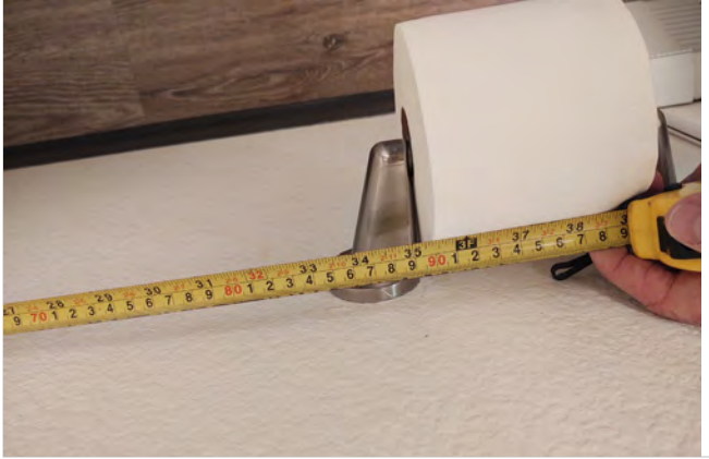
Photo AM9 – Dwelling Unit #115 – Measured distance of toilet paper dispenser exceeds 36” to far edge.
