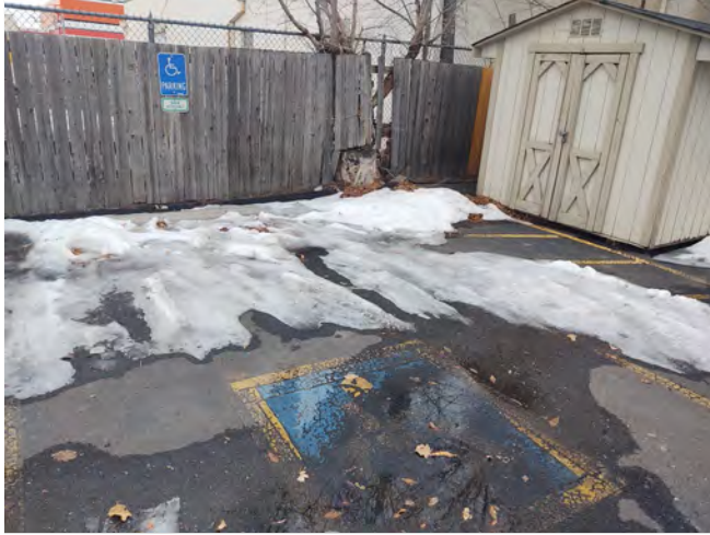
Photo B1 – Accessible parking space and adjacent access aisle.
