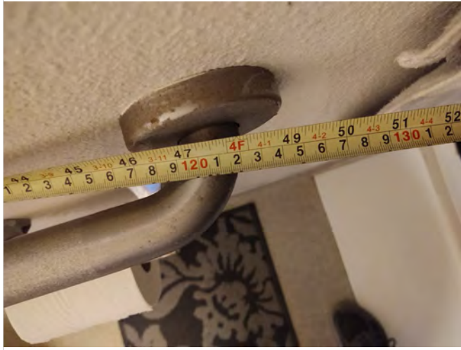
Photo B13 – Dwelling Unit #104 - Measured far end of the side wall grab bar is 47” from the back wall.
