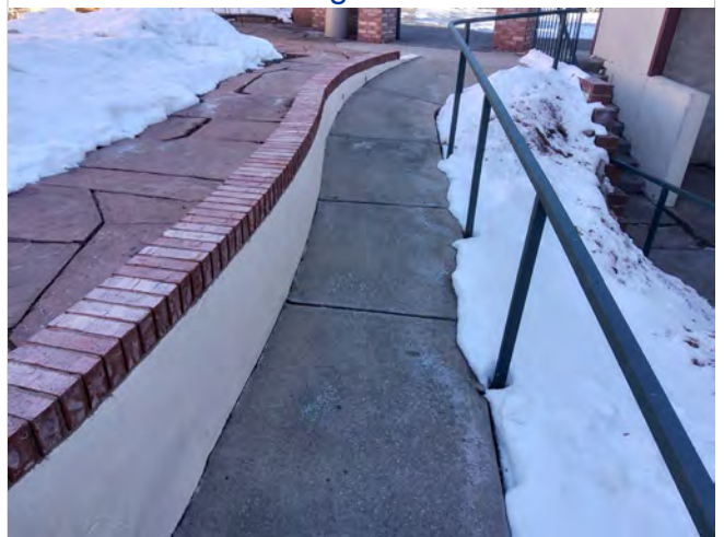
Photo B4 – Ramp at Accessible Route to lower level of dwelling units.
