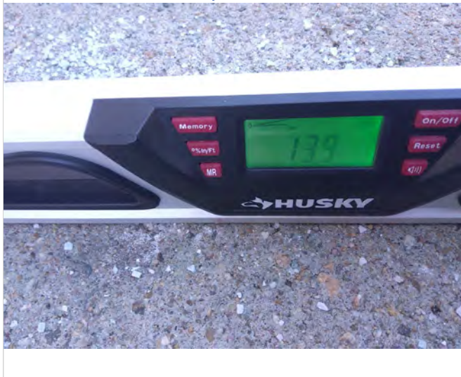
Photo B5 – Measured running slope of accessible route ramp is 13.9%
