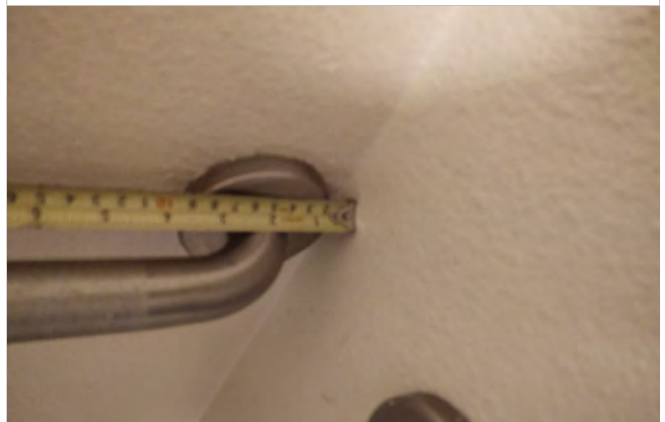
Photo B14 – Dwelling Unit #104 - Measured near end of the rear wall grab bar is 2” from the side wall.
