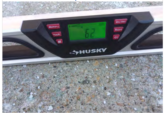
Photo B6 – Measured cross slope of accessible route ramp is 6.2%
