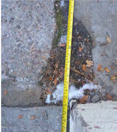
Photo B9 – Measured length of landing at the bottom of the accessible route ramp is 44.”
