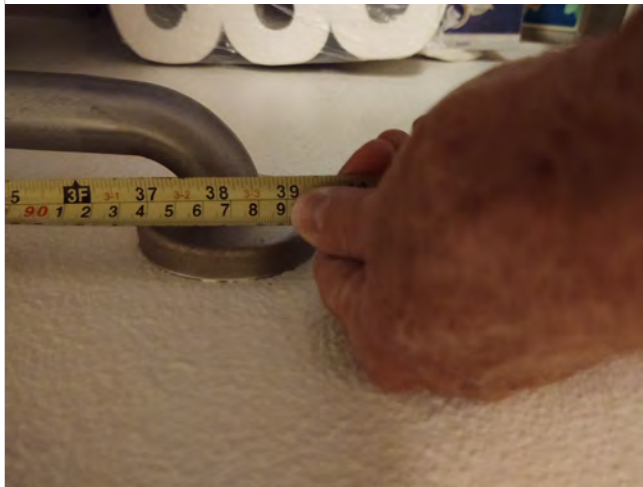
Photo B15 – Dwelling Unit #104 - Measured far end of the rear wall grab bar is 38” from the side wall.
