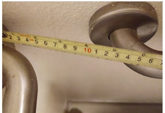
Photo B12 – Dwelling Unit #104 - Measured near end of the side wall grab bar is 5” from the back wall.
