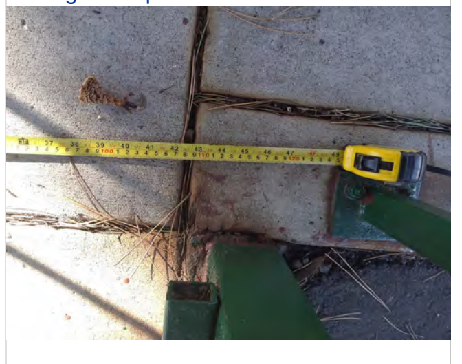
Photo CL4 – Measured width of 43” at bottom landing of ramp.
