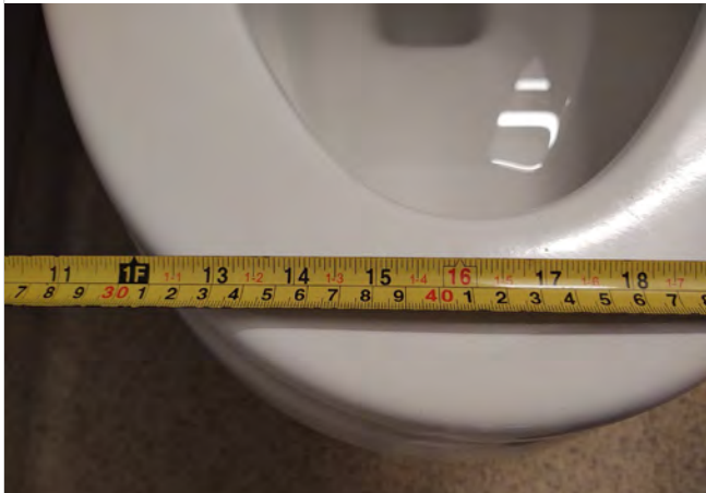
Photo CL7 – Unisex Toilet Room – Measured dimension of 16 ½” to centerline of water closet.
