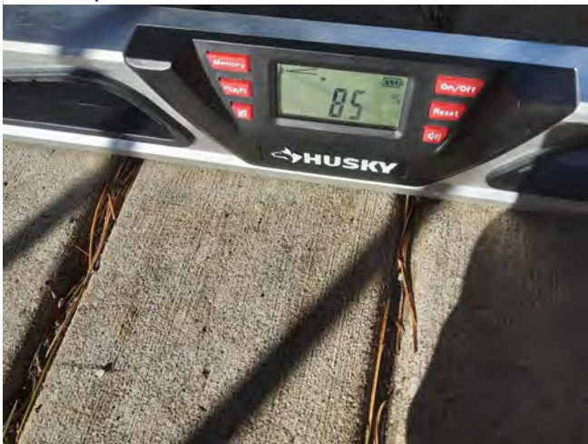
Photo CL3 – Measured running slope of 8.5% on ramp.
