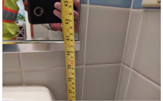
Photo CL6 – Unisex Toilet Room – Measured height of 41” to bottom of reflective edge of mirror.
